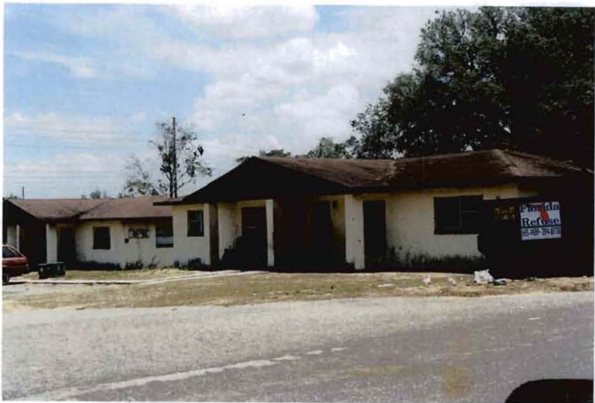
Deteriorated Building & Site.
