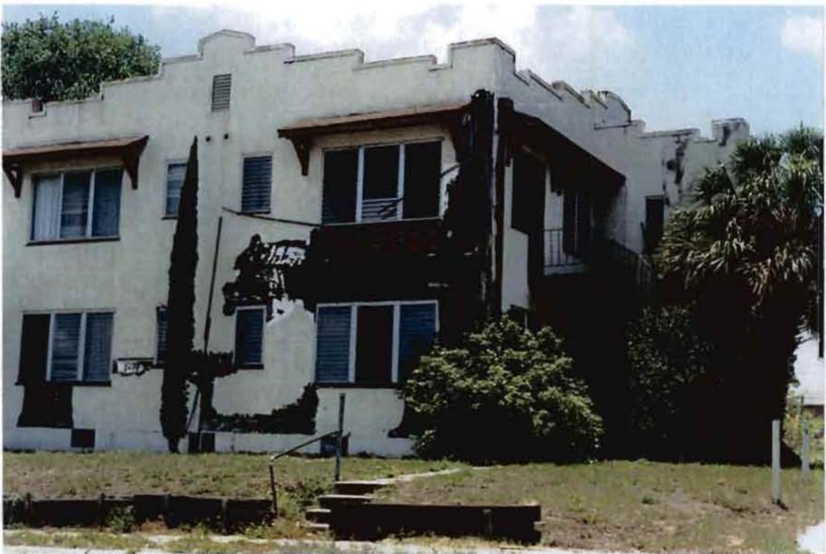
Deteriorated Building & Site.
