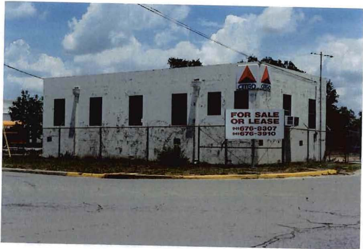
Faulty Accessibility/Usefulness & Deteriorated Building & Site.
