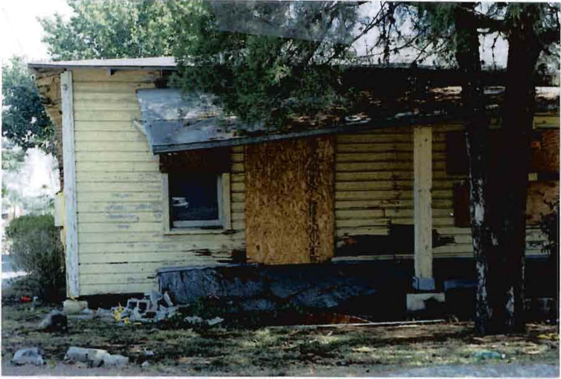
Deteriorated Building & Site.
