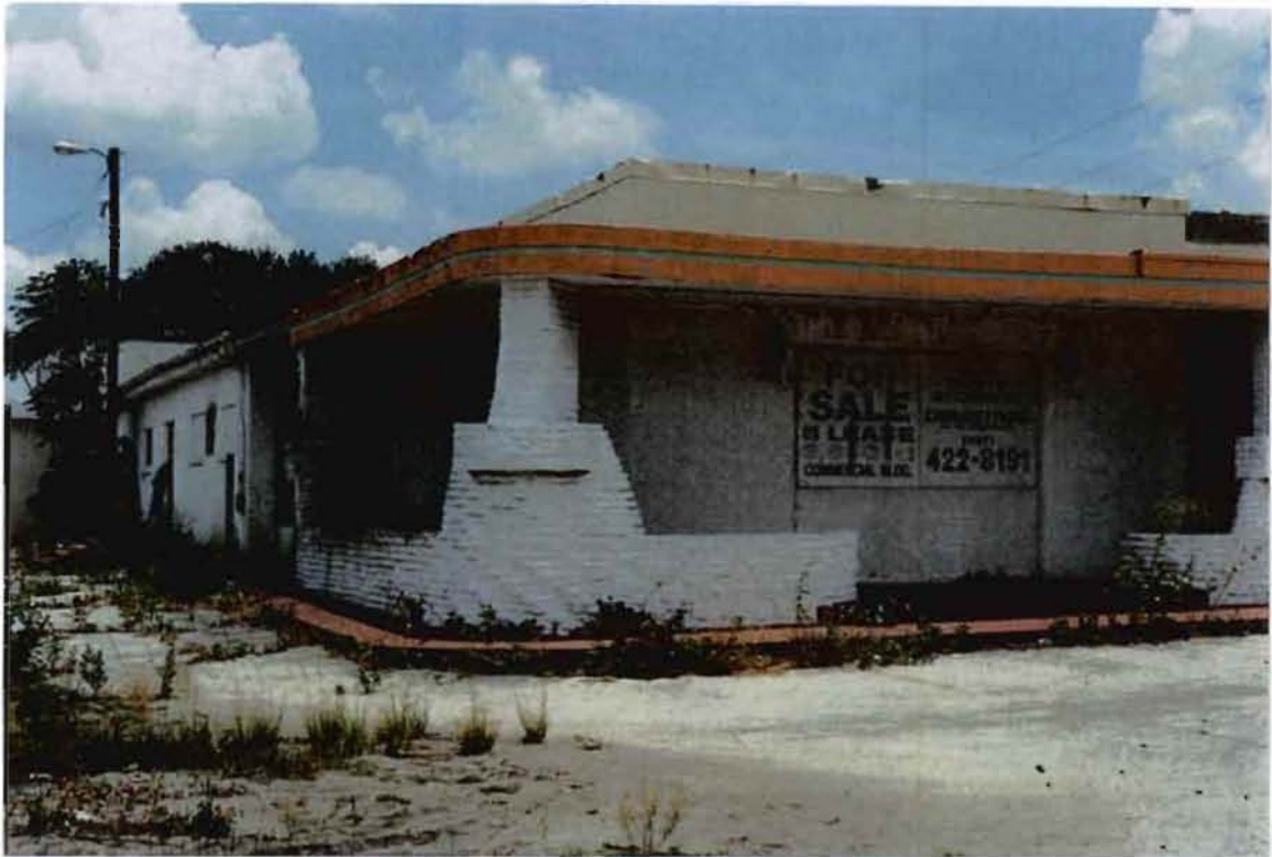
Defective Street Layout, Faulty Accessibility/Usefulness, Unsafe Conditions, Deteriorated Building & Site, and Deteriorated or Hazardous Conditions.
