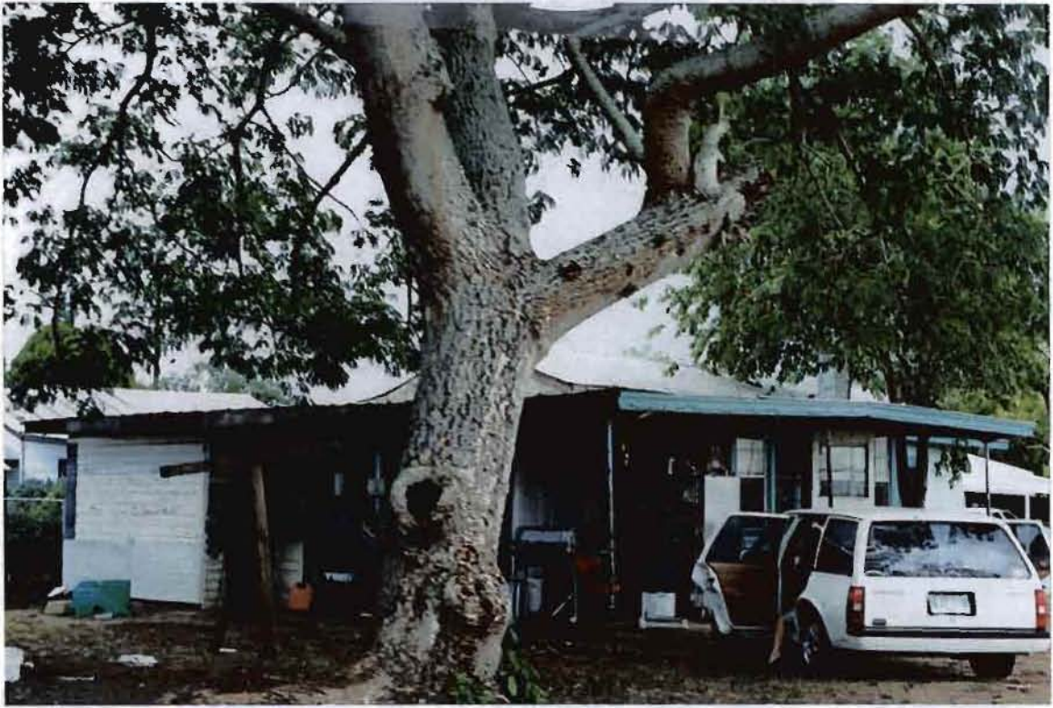
Deteriorated Building & Site.
