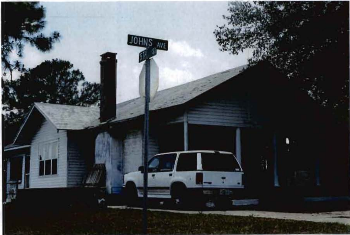
Deteriorated Building & Site.
