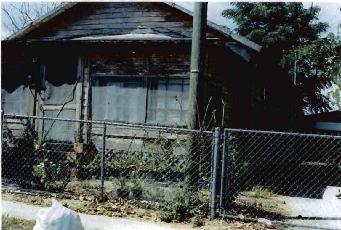
Deteriorated Building & Site.
