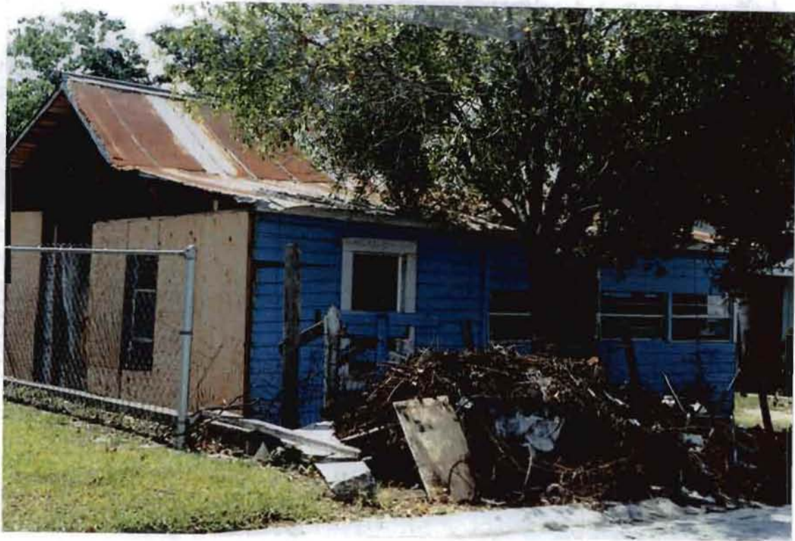
Deteriorated Building & Site.
