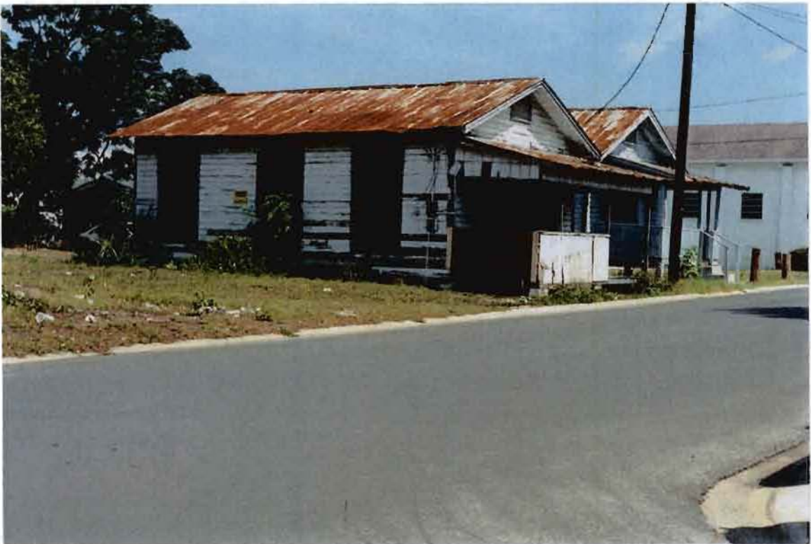
Deteriorated Building & Site.
