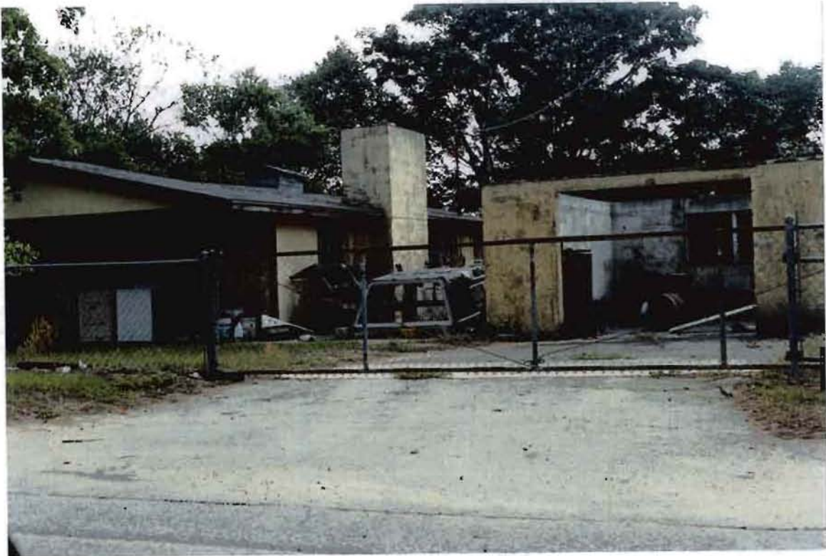
Deteriorated Building & Site.
