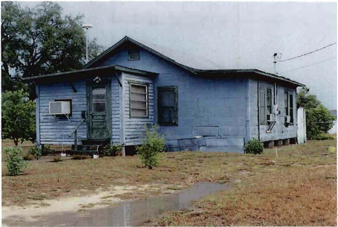
Deteriorated Building & Site.
