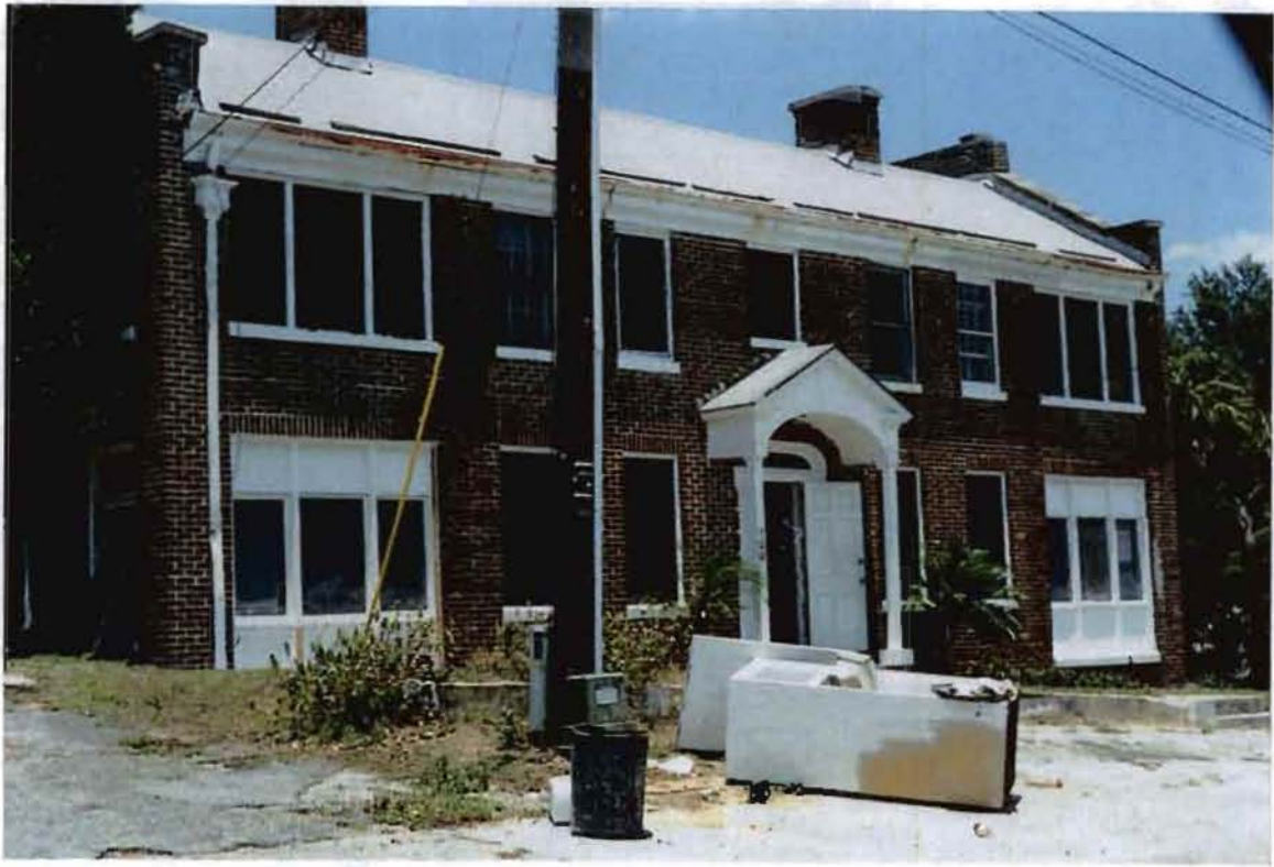
Deteriorated Building & Site.
